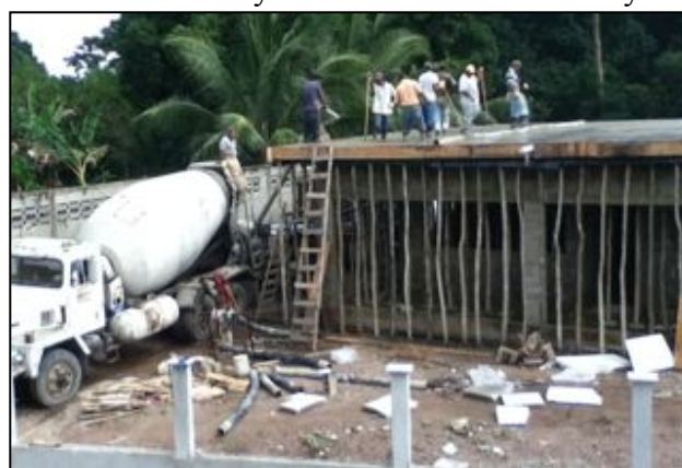
The roof being poured on our new health clinic in Armenia Bonito.
