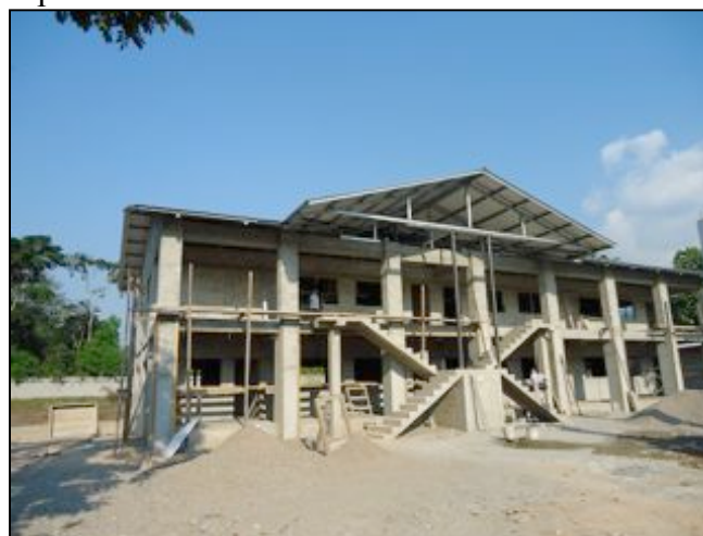
The high school we are building in Armenia Bonito now has a roof.
